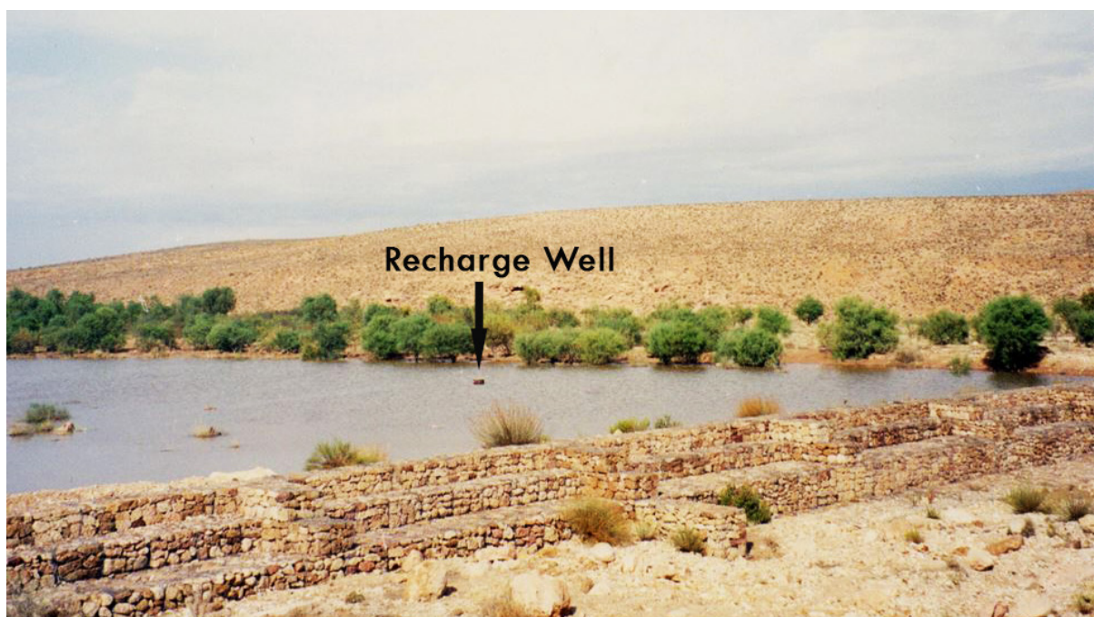
A gabion check dam with a recharge well, Medenine. (Image courtesy: Mohammed Ouessar, IRA)
