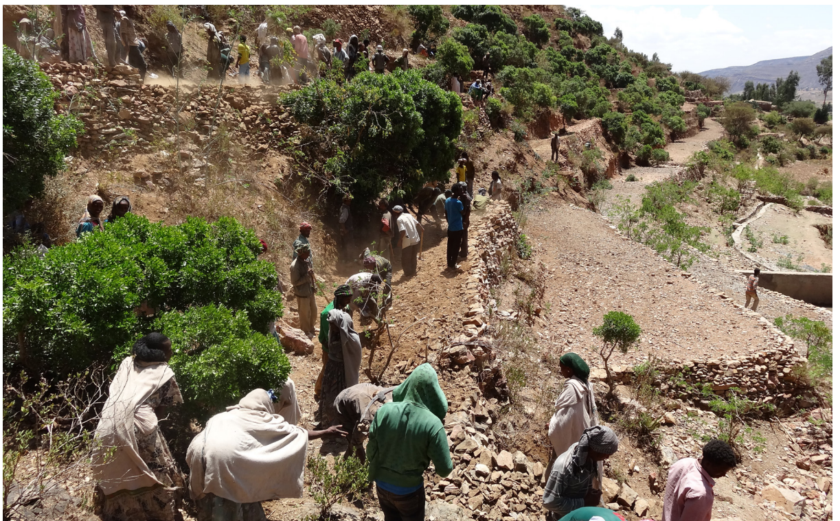
Local community members working on construction of a set of Bench Terraces in Tigray, Ethiopia, during a mass mobilization campaign. (Image Courtesy: Dr. Kifle Woldearegay, Mekelle University)
