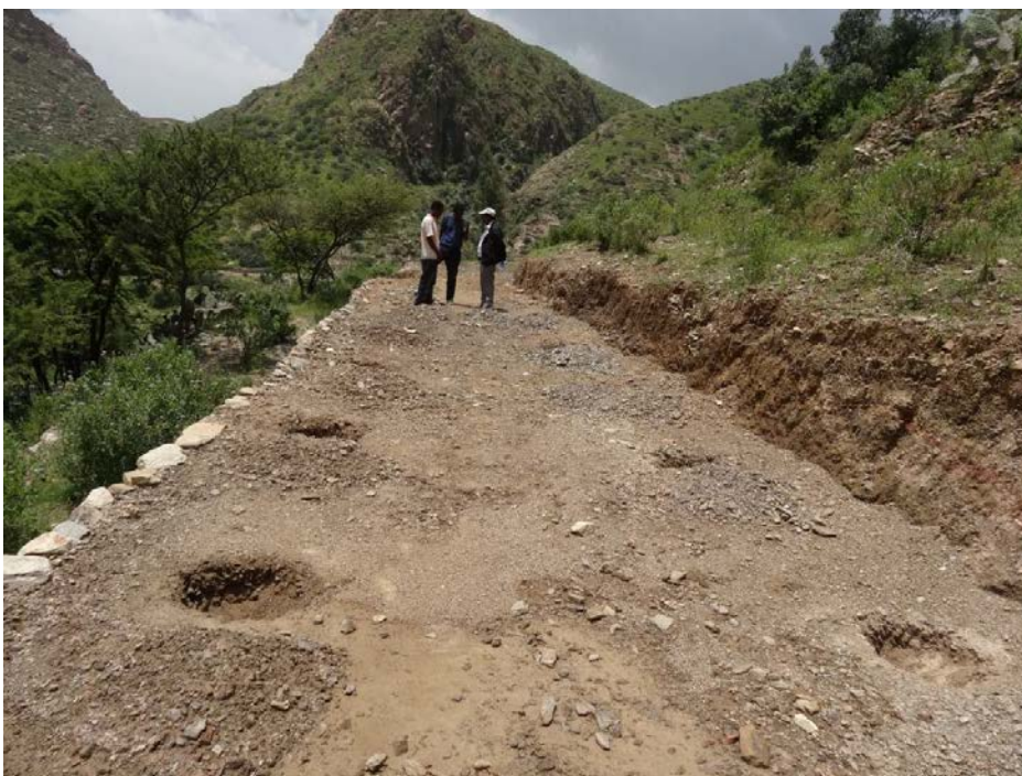
Plate 8. A bench terrace constructed as a demonstration in Gule watershed (funded by Wukro Saint Mary College).
