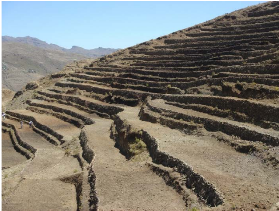
Plate 7. The first bench terrace constructed in Zata watershed in Tigray, Ethiopia (implemented by Tigray Bureau of Agriculture and Rural Development in the year early 2013) (Photo: Kifle Woldearegay).
