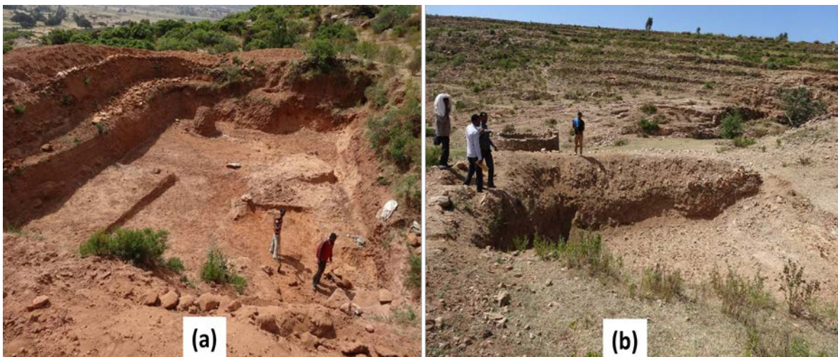
Plate 2. Percolation ponds: (a) 20m long, 15m wide and 2.5m deep, and (b) 12m long, 8m wide and 2m deep constructed to enhance spring discharge and shallow groundwater recharges, Ethiopia.
