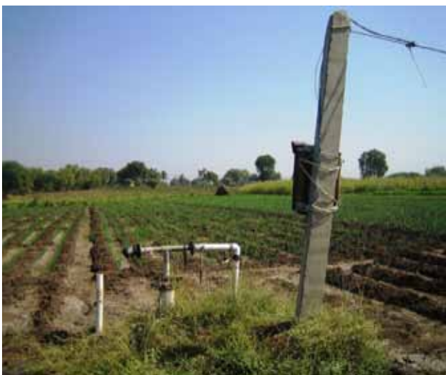
Figure 5 and 6. Dug-well (upper) and tube-well (below) in ICA on left bank, India (Photo credit: Olaf Verheijen)
