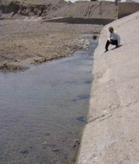
Figure 3. Water emerging from weepholes
