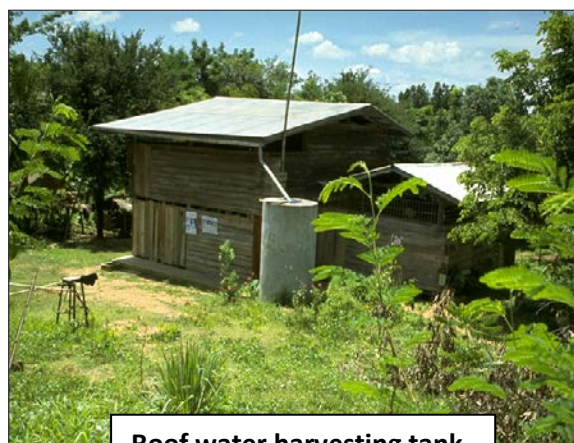
Roof water harvesting tank
